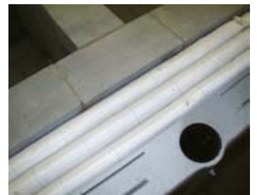
Special bricks in furnace chamber, multi-layered back-up insulation
