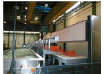
Moving furnace table and material under the C hook of the crane
