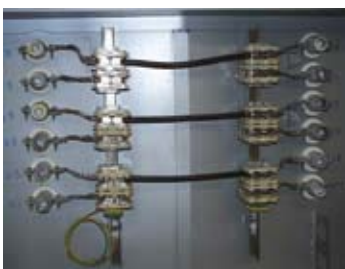
Wiring of the heating elements in sections above each other
