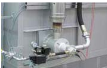
Gas burner firing into a radiant tube
