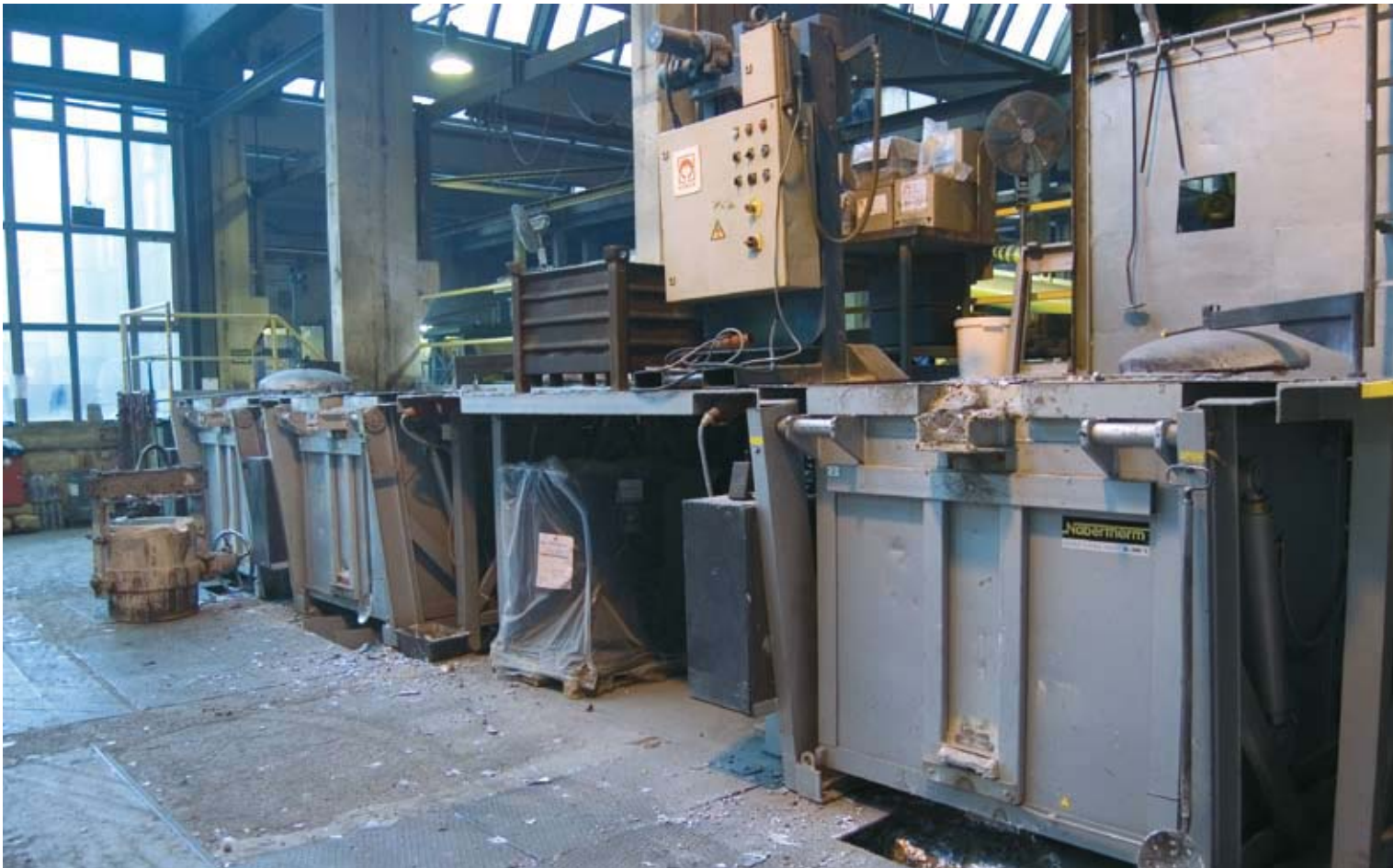
3 x K 300/12 with work platform for melting of aluminum
