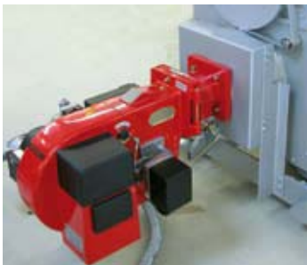
Two-stage burner, fixed on furnace frame
